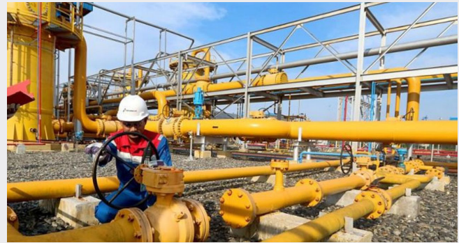
MRS Pertamina Gas Project Indonesia / PT Pertamina Gas
