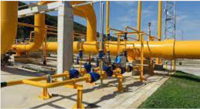
Reconstruction of Gas Pipeline 'Vratsa' 1 in the Section Between BVS 4 and UGS 'Chiren' Bulgaria / Bulgartransgaz
