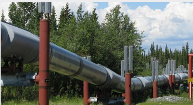
North Macedonia Natural Gas Pipeline Project Macedonia / Hellenic Gas Transmission System Operator (D.E.S.F.A.)
