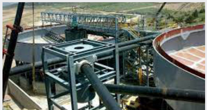
Silver Mineral Processing Plant Mud and Water Line
