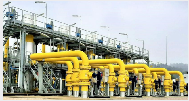
Connecting Gas Pipe Line Poland/ Slovakia Compressor Station PJ161.2 - Filtration Slovakia / Eustream
